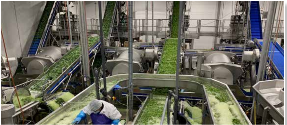
Leafy vegetable processing line including externally purchased packaging system. This line is completely customer specific and has been designed based on the customer's preferences and requirements.
